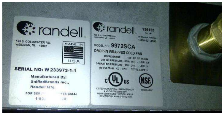
Located on underside of unit near drain.
