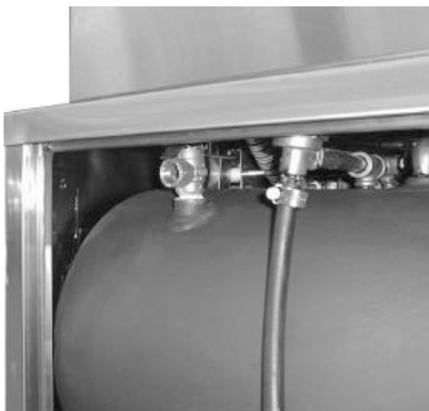
One of the pressure relief safety valves is located on the top left rear of the boiler.
