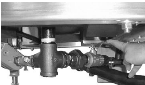
The manual drain valve is located under the boiler.
