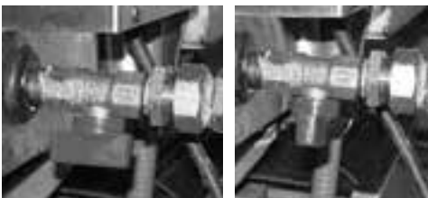
Gas valve "On"
