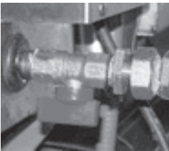
Gas valve "On"
