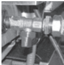
Gas valve "Off"
